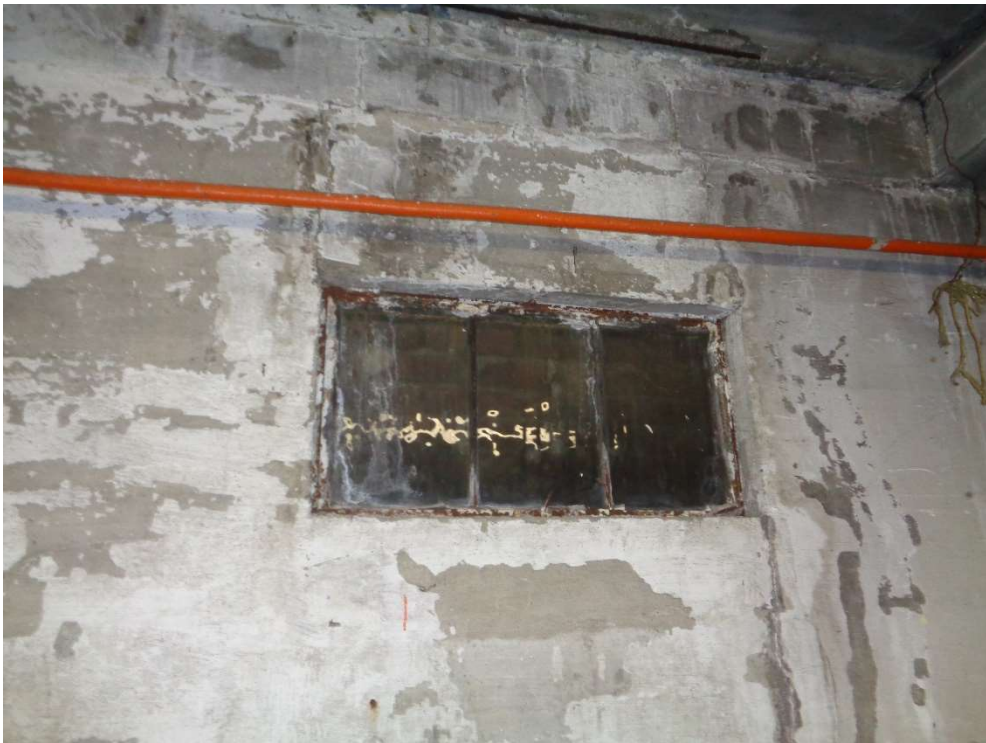
Photo of the ACM window glazing located on the rear window of bay 2 area. (CAC23218-02)
