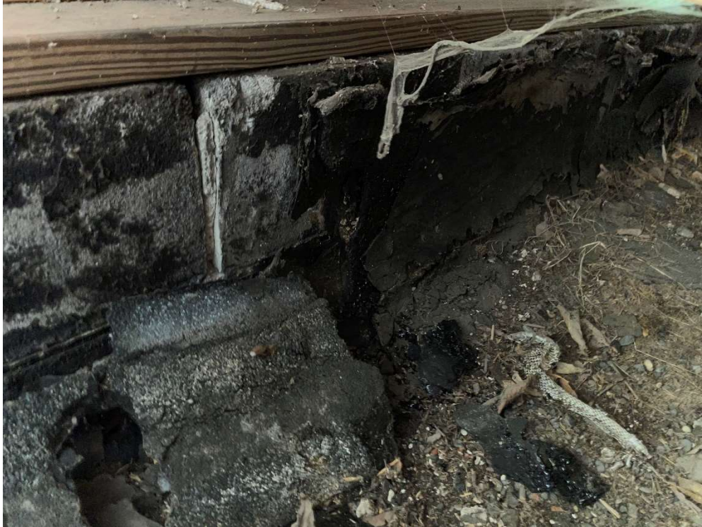
Photo of the ACM black flashing on the parapet wall of the original roof located under the metal roof. (CAC23218-11)
