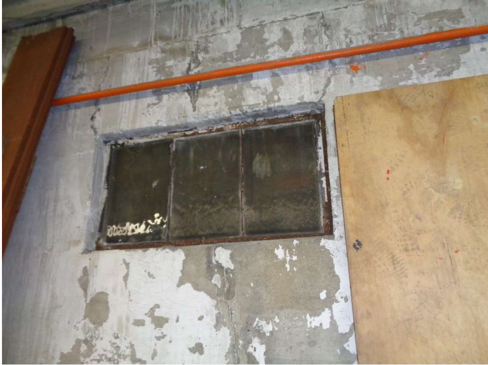
Photo of the ACM window glazing located on the rear window of bay 2 area. (CAC23218-01)
